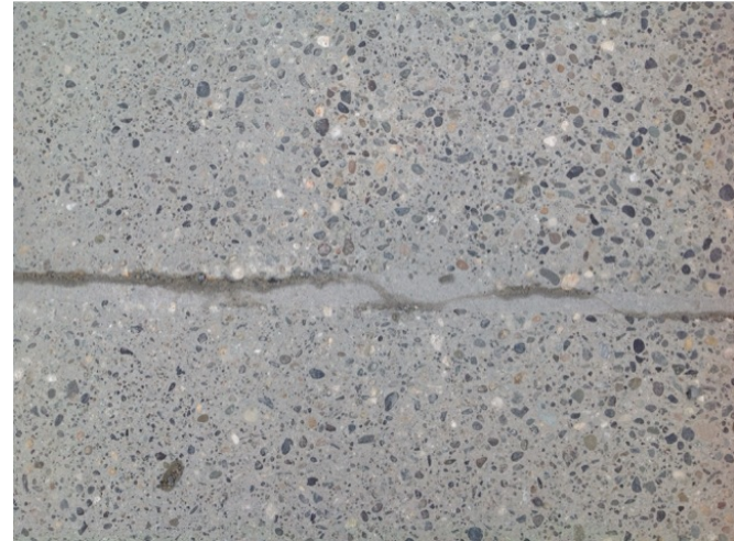
cracks in deck joints
